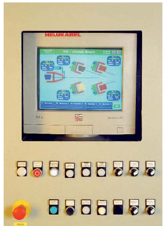
Standardised process control and visualisation of an extrusion system at our Windsbach factory.
